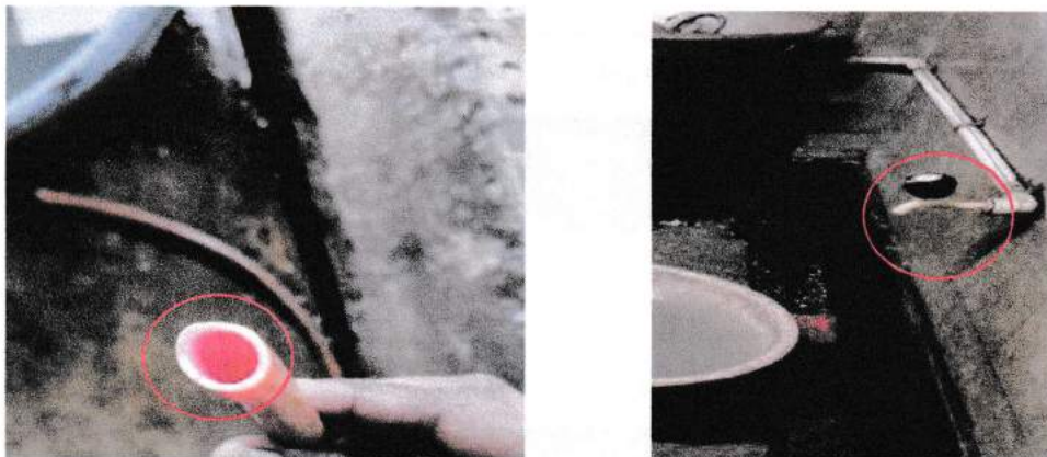
Figure 5. Taps photos in institution
