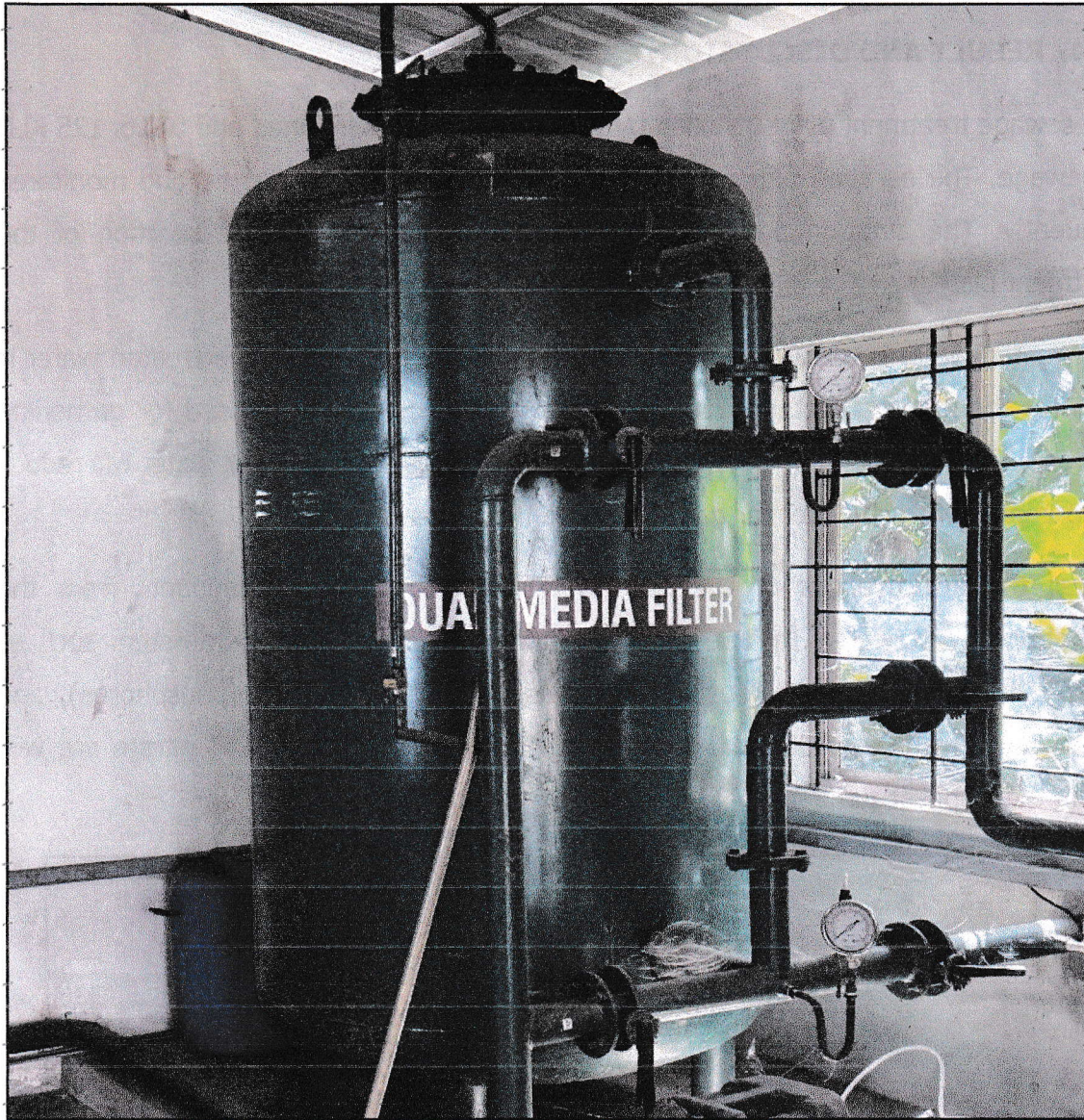
Figure 4: Filtration unit at SMVITM
