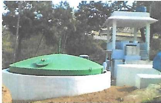
Fig. 3.2 : Bio – Gas Plant
